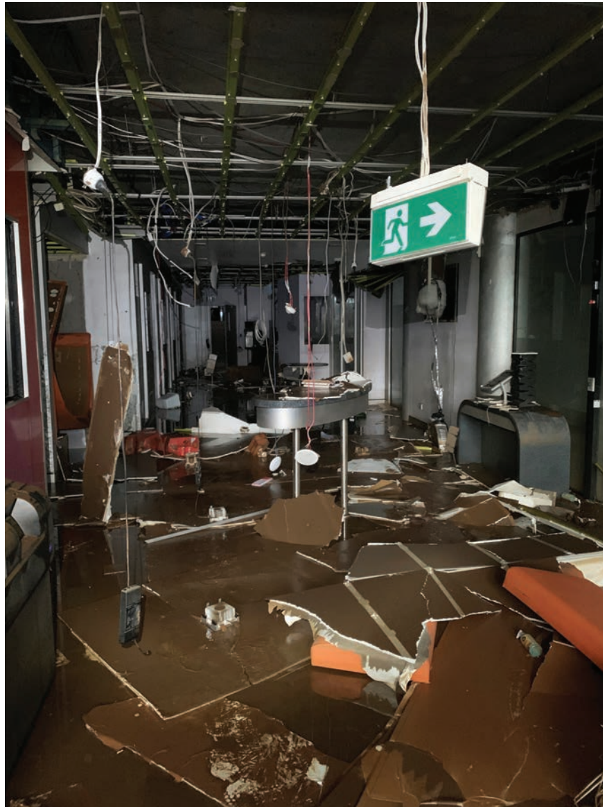
Flood damage at Lismore branch and head office, Molesworth Street
